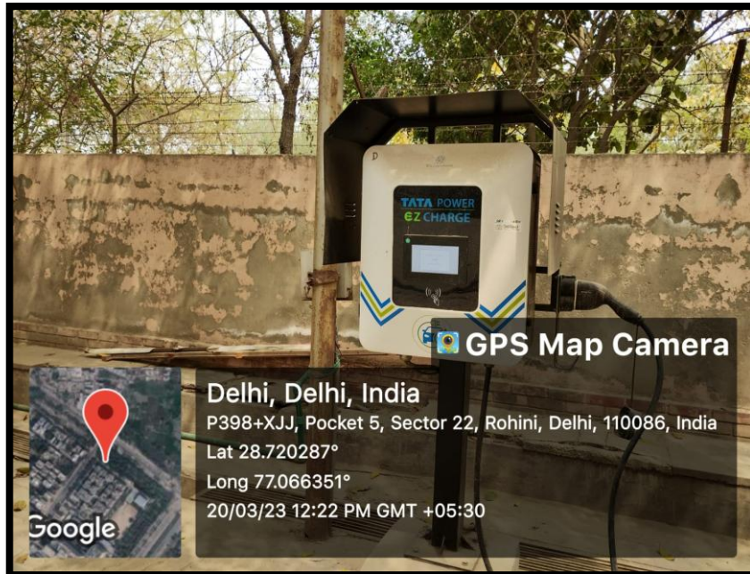
Electric Vehicle Charging Point in the Institute
