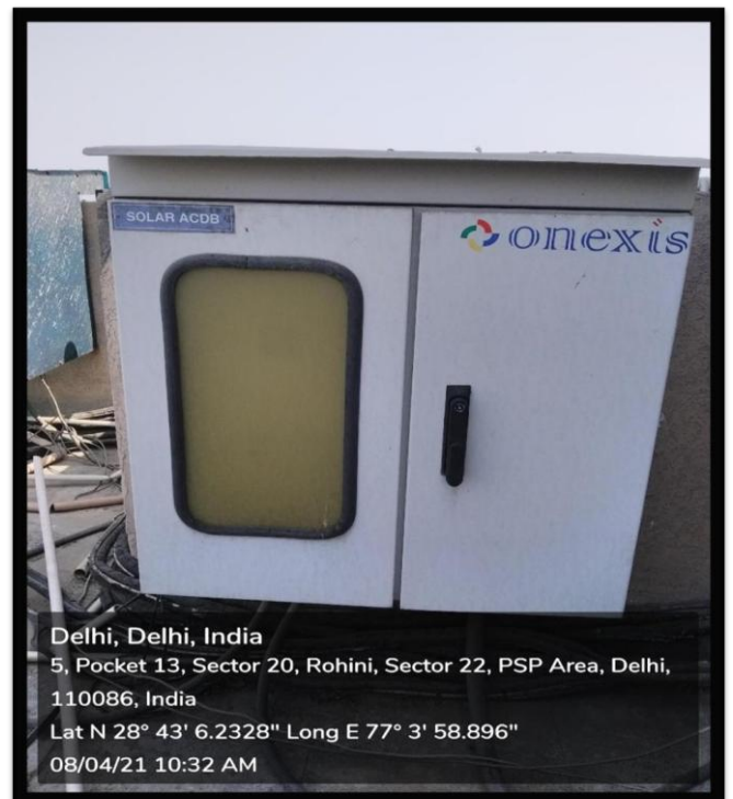
Photo-4: Solar Panel Box
