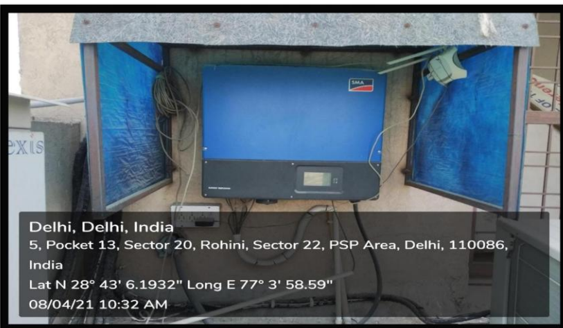
Photo-3: Controller of the Solar Panel
