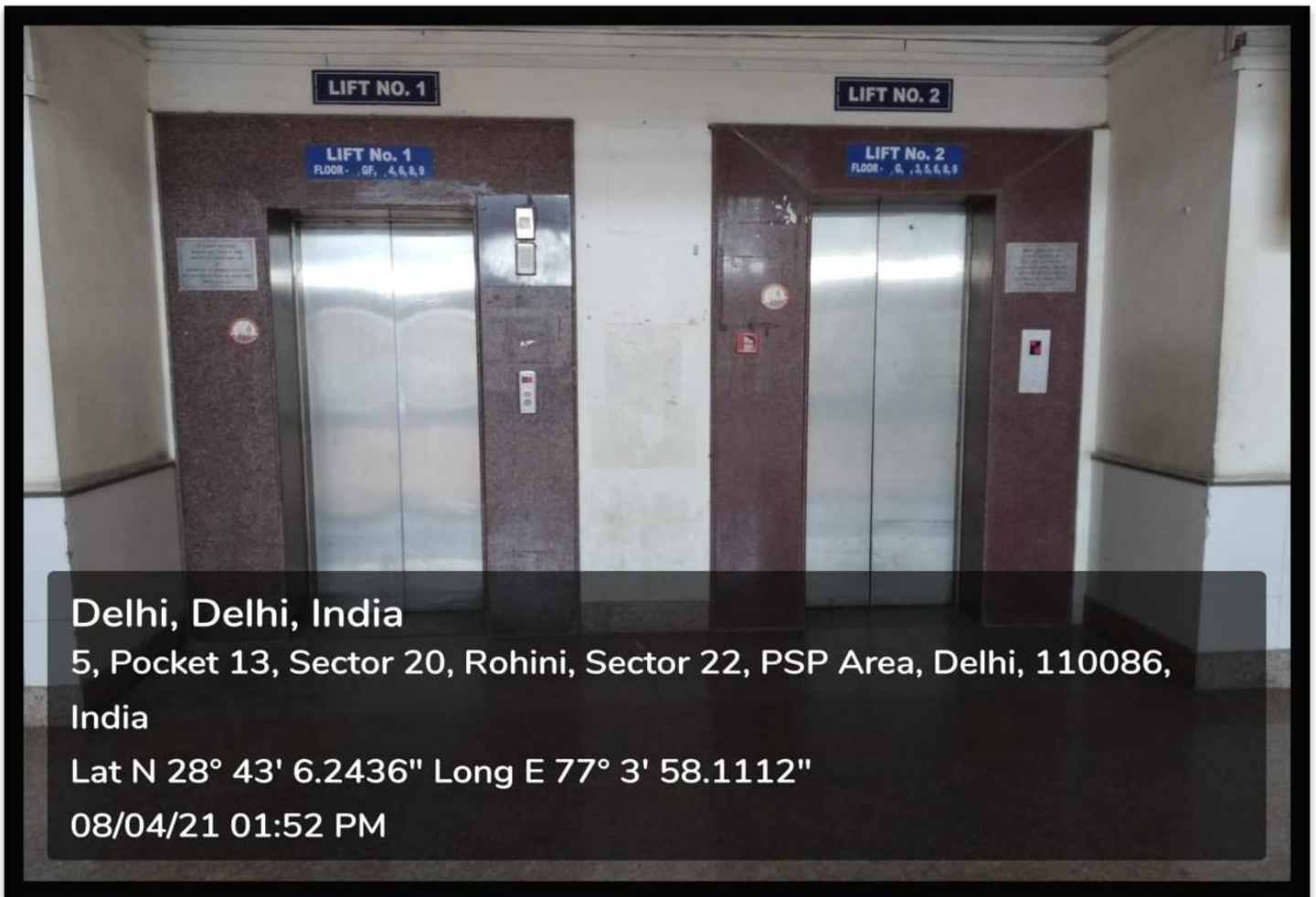
Lift in the Building of the Institution
