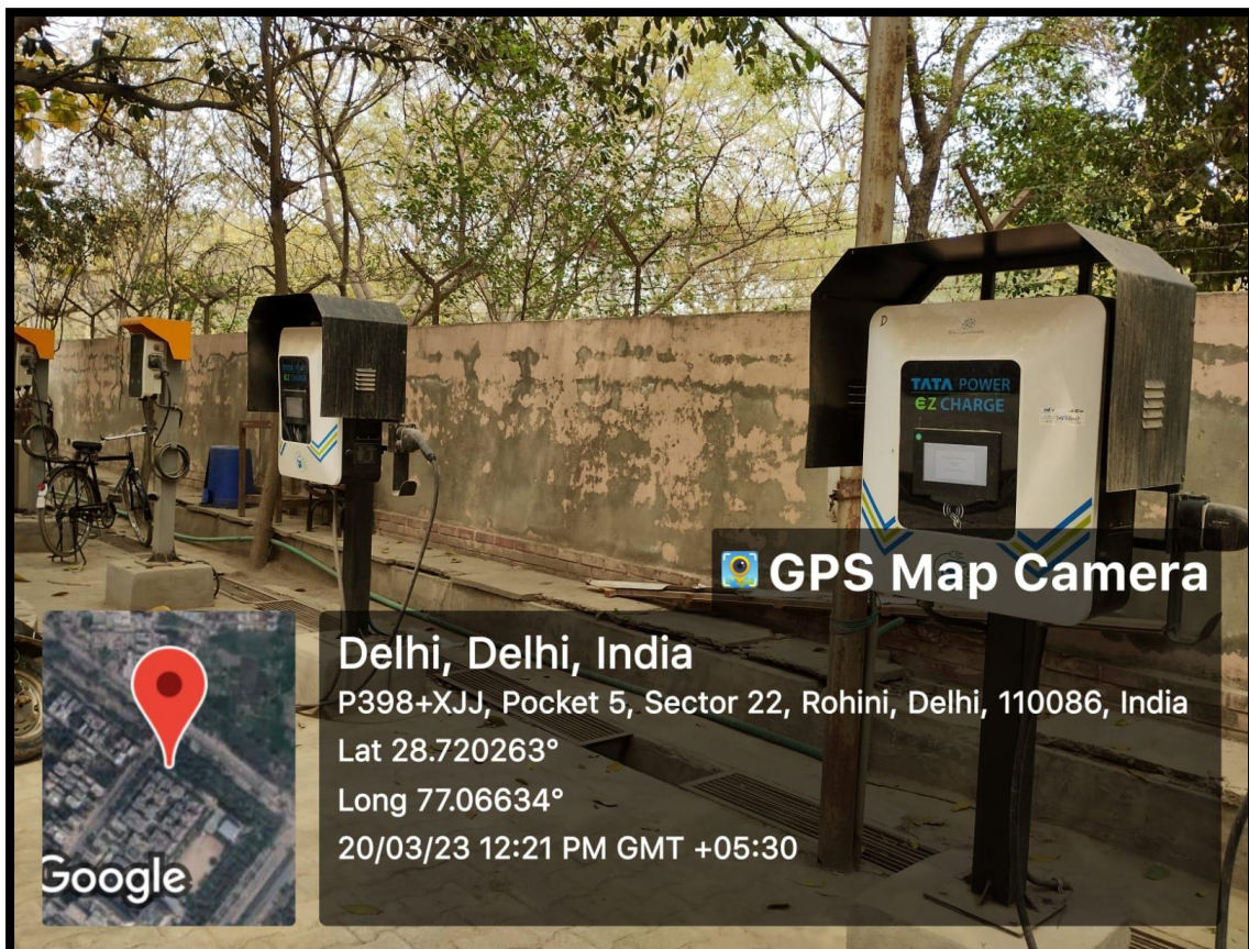
Electric Vehicle Charging Station in the Institute
